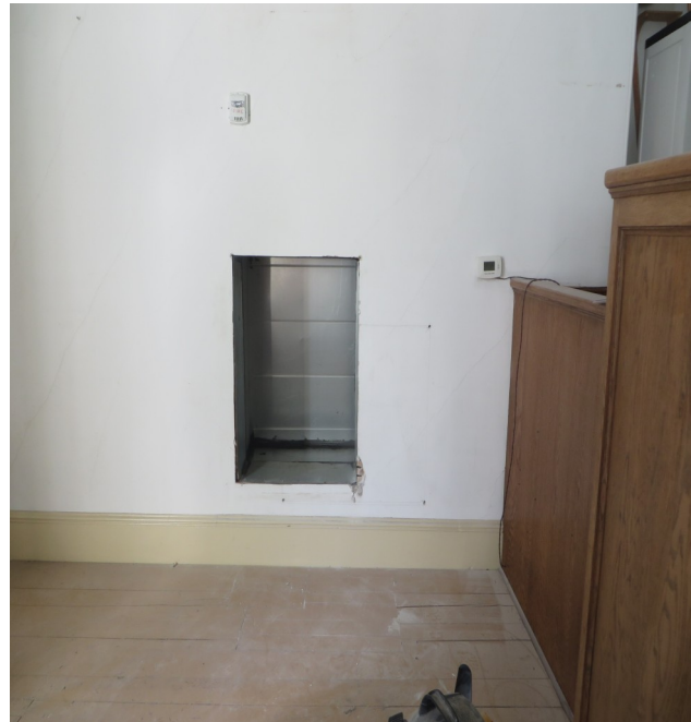
Cold air duct work in sanctuary
