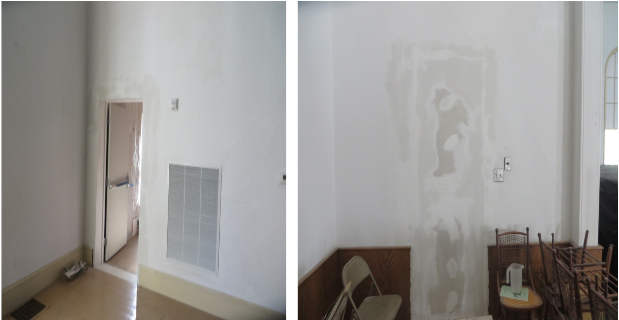
Sanctuary with a new door opening and an old door sealed off
